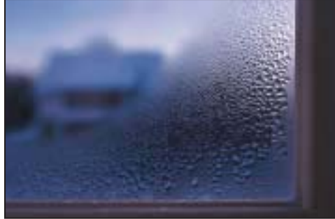
Condensation on the inside of a windowpane.
